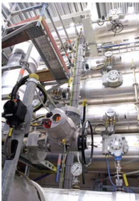
The circuit for gas meters utilises Rotork IQ and IQT intelligent electric actuators.
