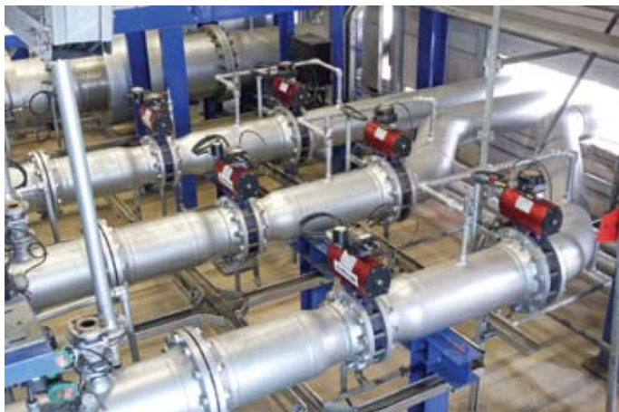
Consisting of three circulation systems, the EuroLoop plant for liquid meter calibration requires 43 pneumatic actuators.
