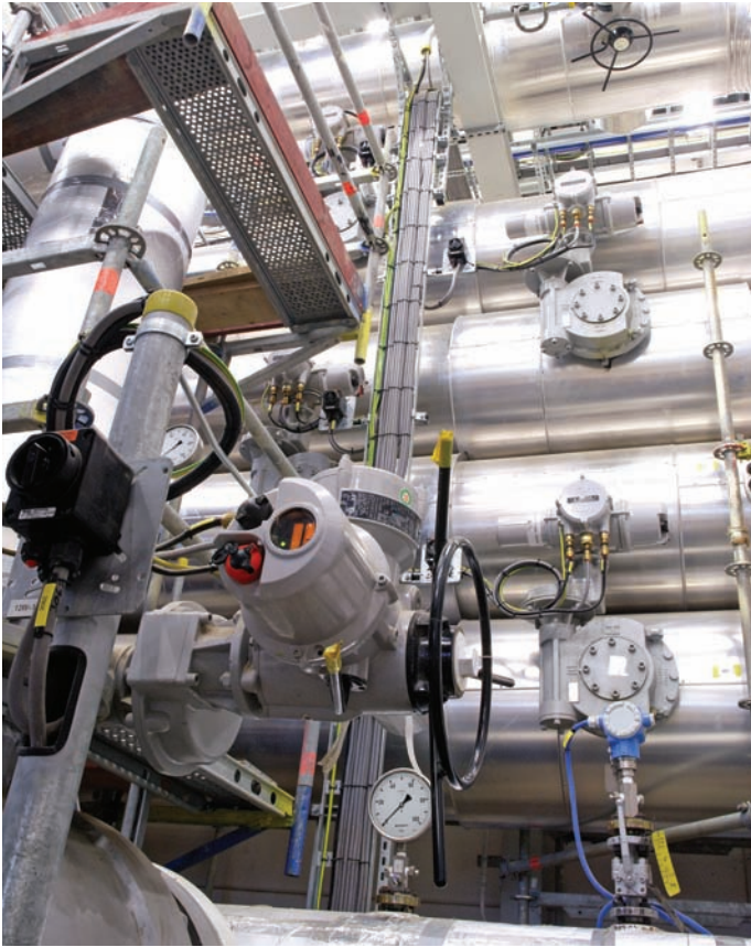
Some of the Rotork RC200 Series pneumatic valve actuator installations on the liquid meter calibration loop at EuroLoop
