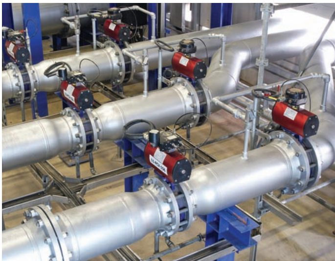
Pakscan-enabled Rotork IQ electric actuators with Rotork Gears IW Range worm gearboxes installed on part of the EuroLoop gas meter calibration circuit
